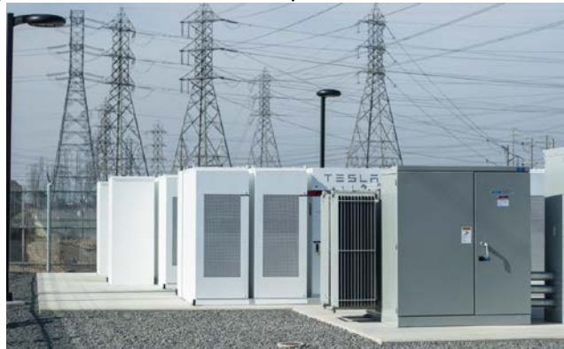
Aliso Canyon Mira Loma Li-ion Battery Jan 2017
